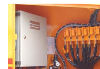
▲electric control panel & control v/v for boom
